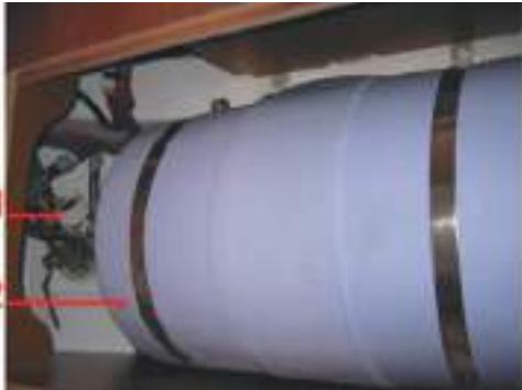
Water heater 220V- Saloon seating Starboard
