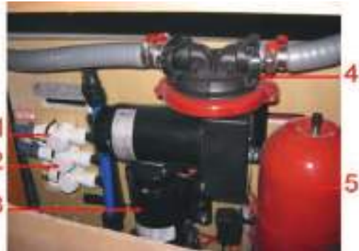
Plumbing board Saloon backrest Starboard
