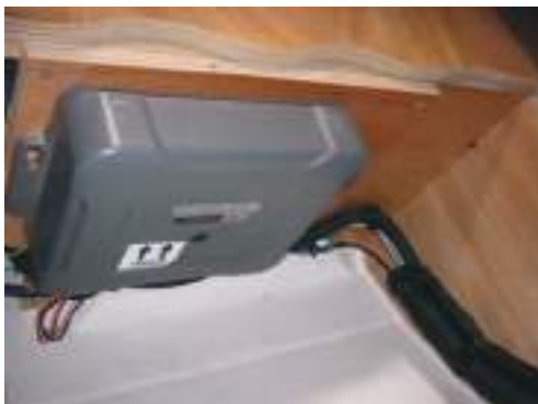
Vessel Management Unit - Bulkhead - Port aft cabin
