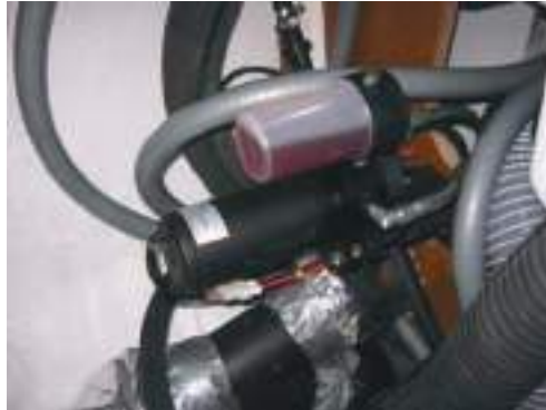
Auto pilot Access: Port cockpit locker
